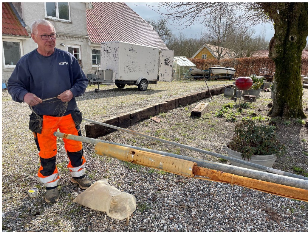
Figure 3. As preparation for the depth specific sampling, the permanent pump must be removed. May 1 st , 2023, DGU 49.386.
