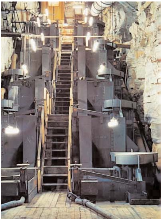
The flotation plant located underground in a 67 x 7 m chamber. Lead and zinc cells are on opposing sides with eleven cells in each circuit. Photo: Bent Sørensen, 'Blyminen i Mesters Vig', published by Atuagkat, 2005.
