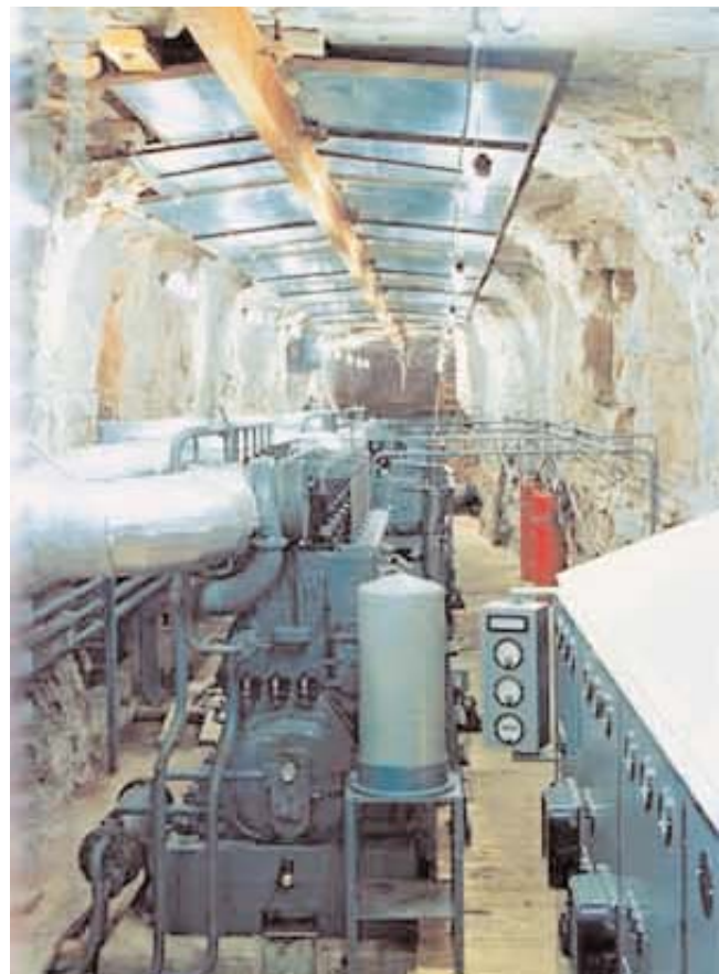
Diesel power plant installed in a 60 m-long rock hall. Photo: Bent Sørensen, 'Blyminen i Mesters Vig', published by Atuagkat, 2005.
